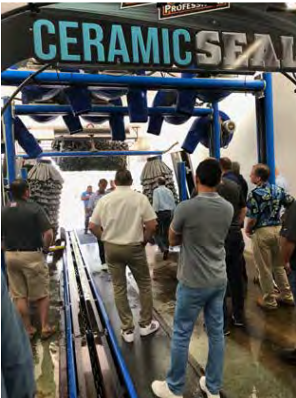
The site boasts a 165-foot conveyor equipped with Motor City/Service One Installer, NCS chemistry and Micrologic controls.
